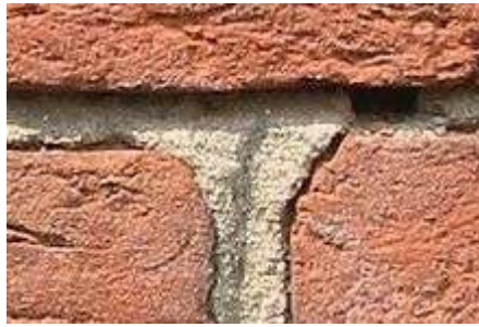
Mortar holding weathered bricks
