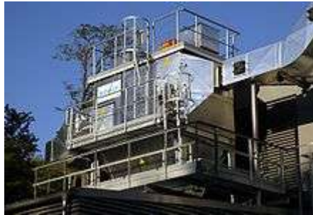
Electrostatic precipitator of a bio mass heating system with a heat power of 2 MW
